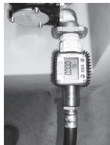
Fig. 6.2.1: Flow meter for 1251 / 2001 tank
