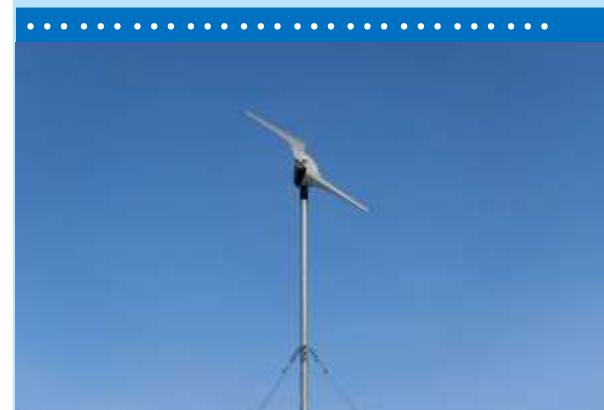
Stand-alone installation on a tower
