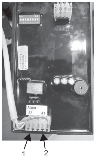
Fig. 4: Cable connection at the control unit
